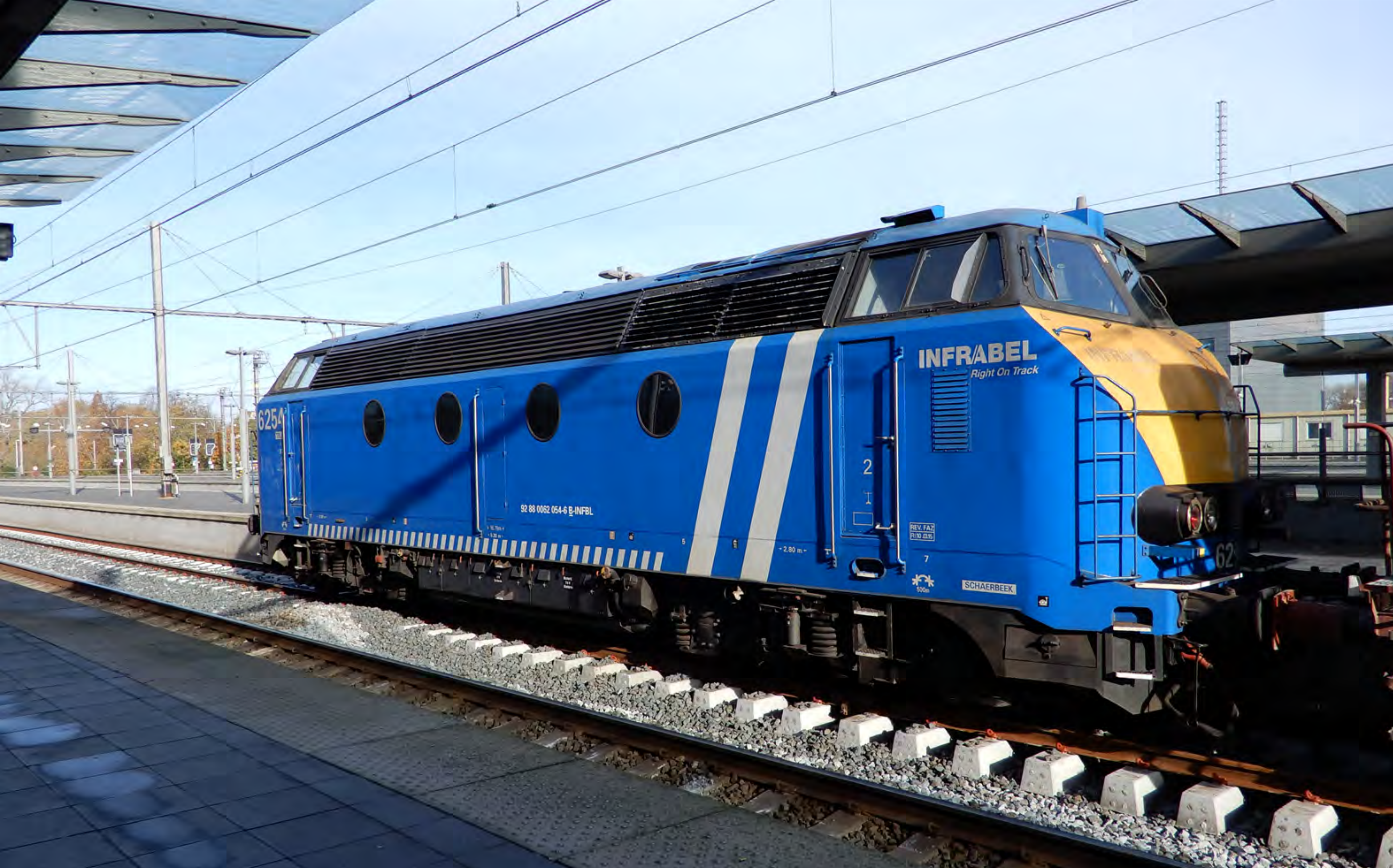
▶ Infrabel BN/ACE Class 62 No. 6254 drops ballast on newly laid track at Brugge on November 14th. Stephen Stepney
