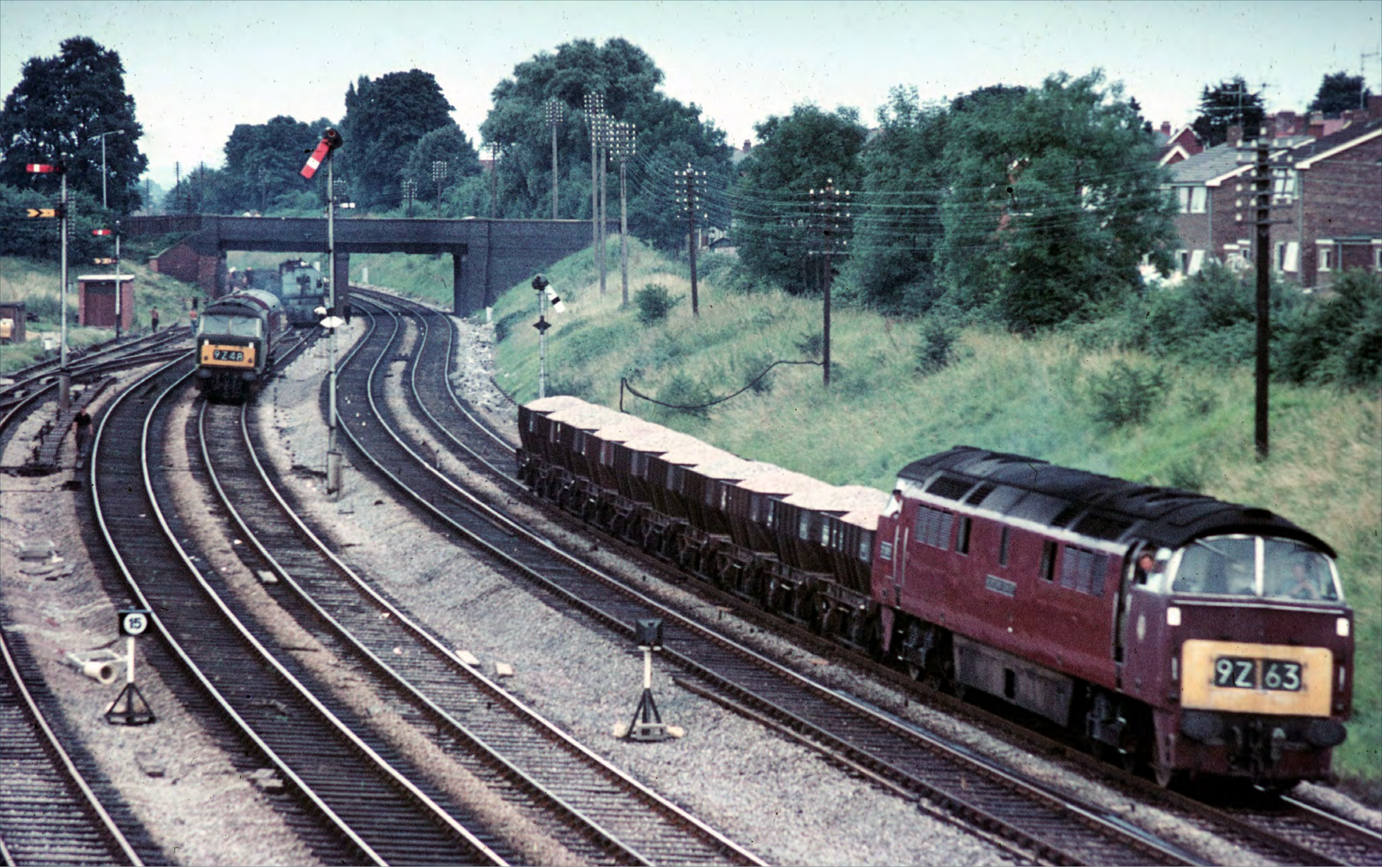
This photo was taken during the remodelling of Tuffley Junction, south of Gloucester, over the May bank holiday weekend in 1968. Track rationalisation took place in conjunction with the reduction from four to two tracks south to Standish Junction. The ex-Midland lines from Eastgate station were slewed across to link up with the ex-GW line, with an improved alignment thus enabling speed limits to be relaxed. Here a 'Hymek' on an engineering train is seen standing on the ex-Midland tracks, whilst a 'Western' heads south on the ex-Western tracks with a ballast train that will return to the site later. Christopher Baldwin
