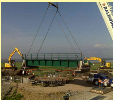
Photos show the old bridge (Top) and the new bridge (Above) ©Network Rail
