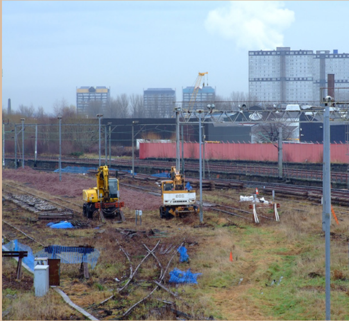
Construction work has finally gone underway for the Shields T.M.D. extension which is part of the G.A.R.L. (Glasgow Airport Rail Link) Project.
