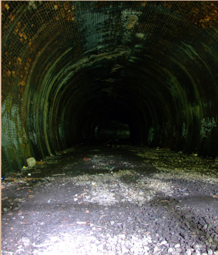
A photograph of the Kirklee tunnel mouth seen from Botanic Gardens train station. The tunnel takes you through to the original Kirklee station which was once a station also owned by the Grand Central Railway which opened on 10th August 1896 and before the station officially closed to passengers and passenger trains between 1st January 1917 and 2nd March 1919. The station was closed due to wartime economy during World War I. Until 6th February 1939 the station was still open and in use to passengers only (not passenger trains) when the train station was fully closed on 5th October 1964.
