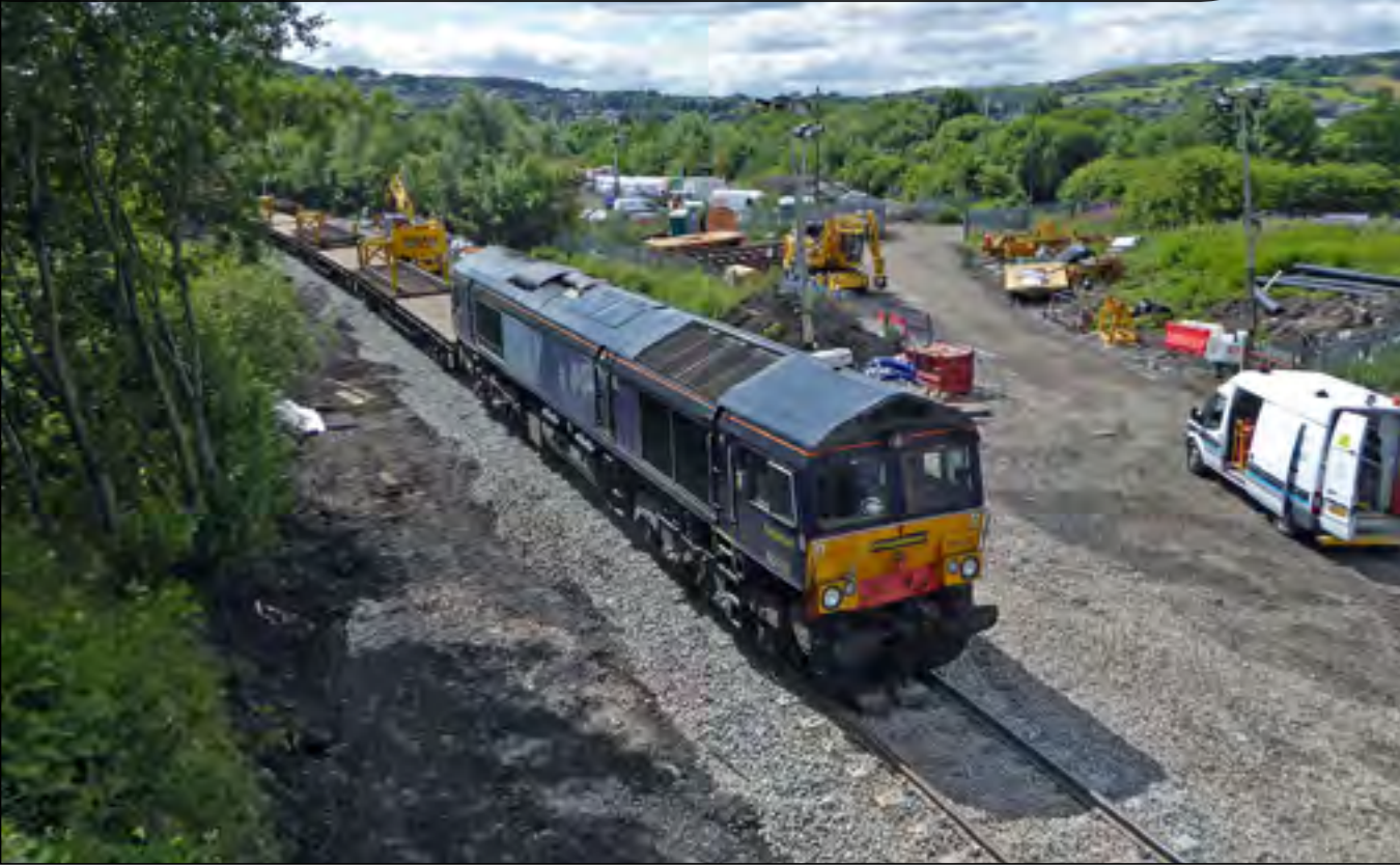
On July 30th, Class 66 419 is seen heading an engineers train at Goose House Lane Darwen in connection with the line improvements between Blackburn and Bolton. Michael Lynam
