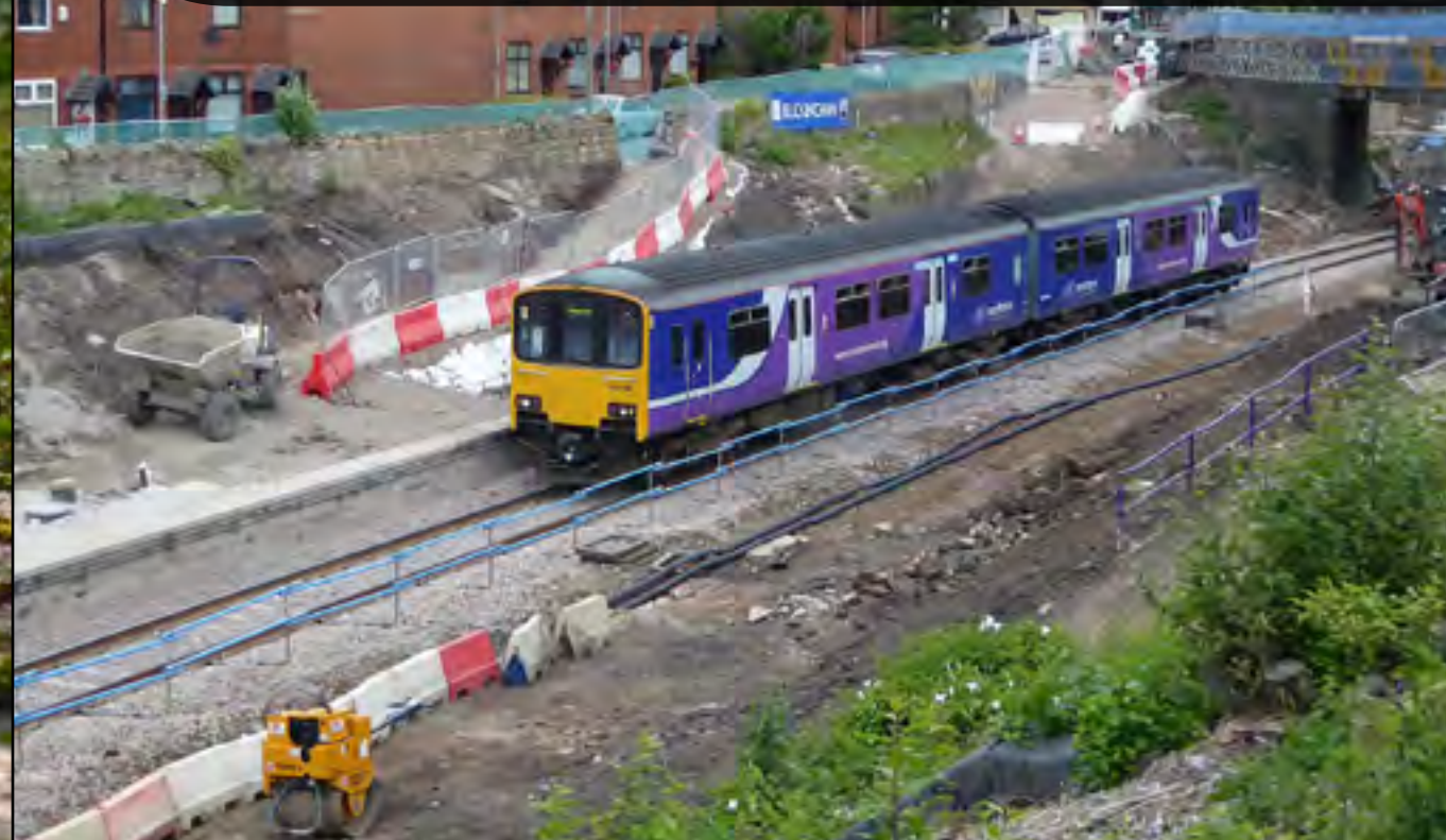
Northern Rail's Class 150 149 passes through a partially rebuilt Farnworth station working a Manchester Victoria - Blackpool North service. Currently the Manchester line through Farnworth Tunnel is being enlarged ready for electrification. Michael Lynam
