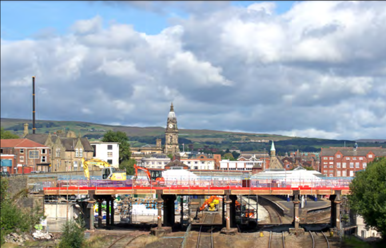
With the skyline of Bolton in the background, work can be seen well advanced for the demolition of Orlando Bridge. Dave Felton
