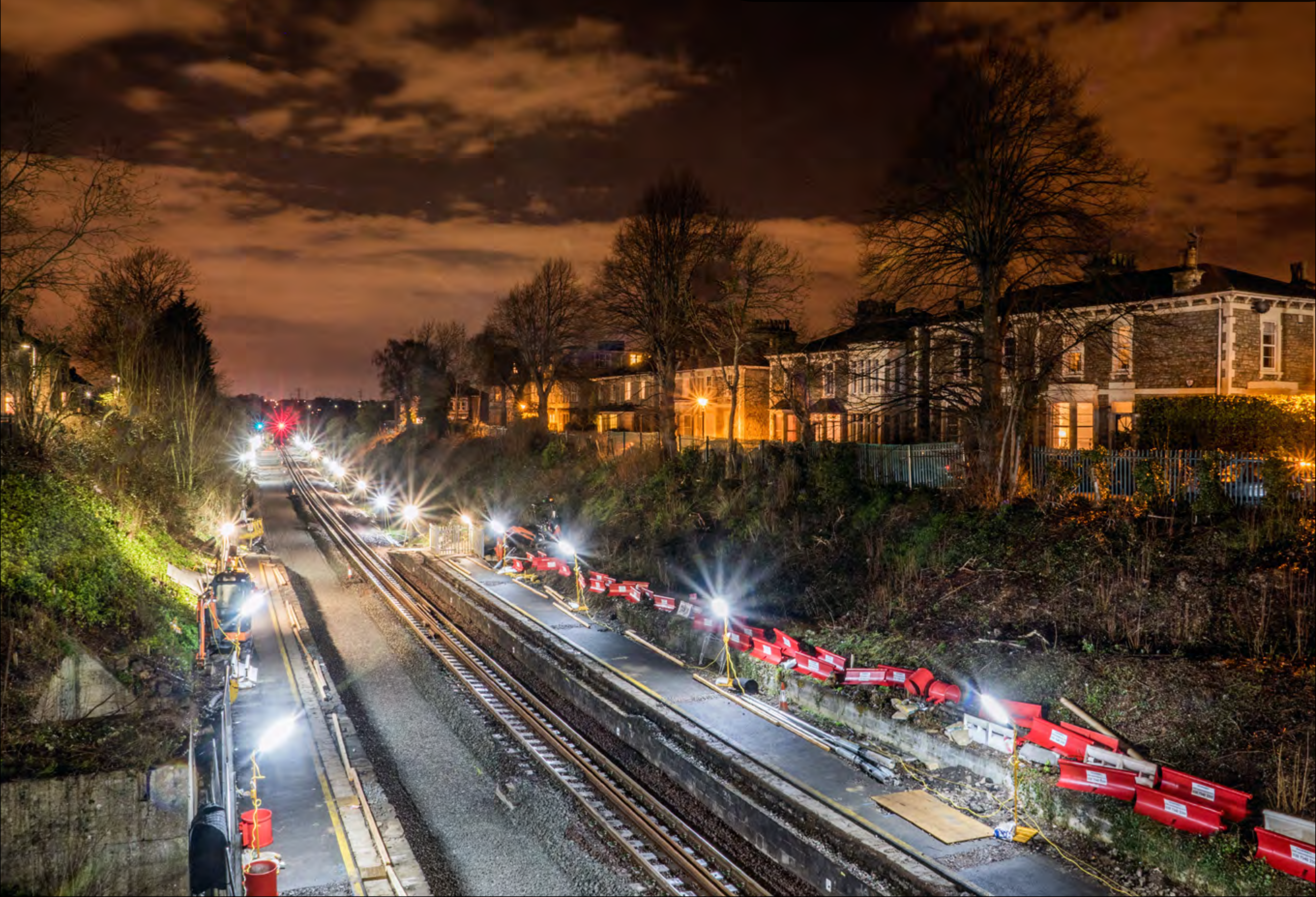
A nocturnal view of the engineering works at Keynsham station taken on April 4th as the line was completely shut between Bath and Bristol for just over a week. Sam Bilner
