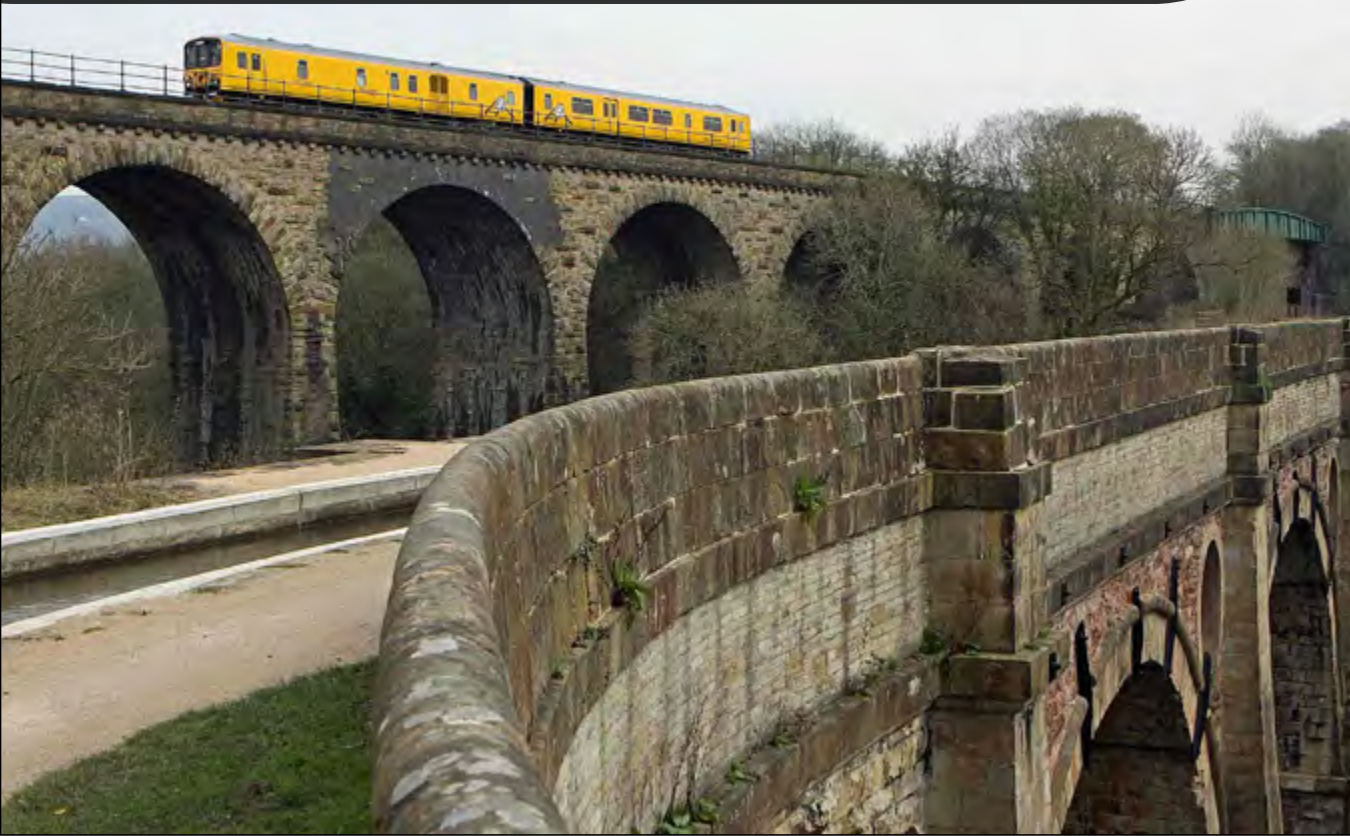
Class 950 001 crosses Marple Viaduct on April 11th with the 06:41 Derby RTC - Longsight. Marple Aqueduct carries the Peak Forest Canal 100 feet above the River Goyt. Nick Clemson
