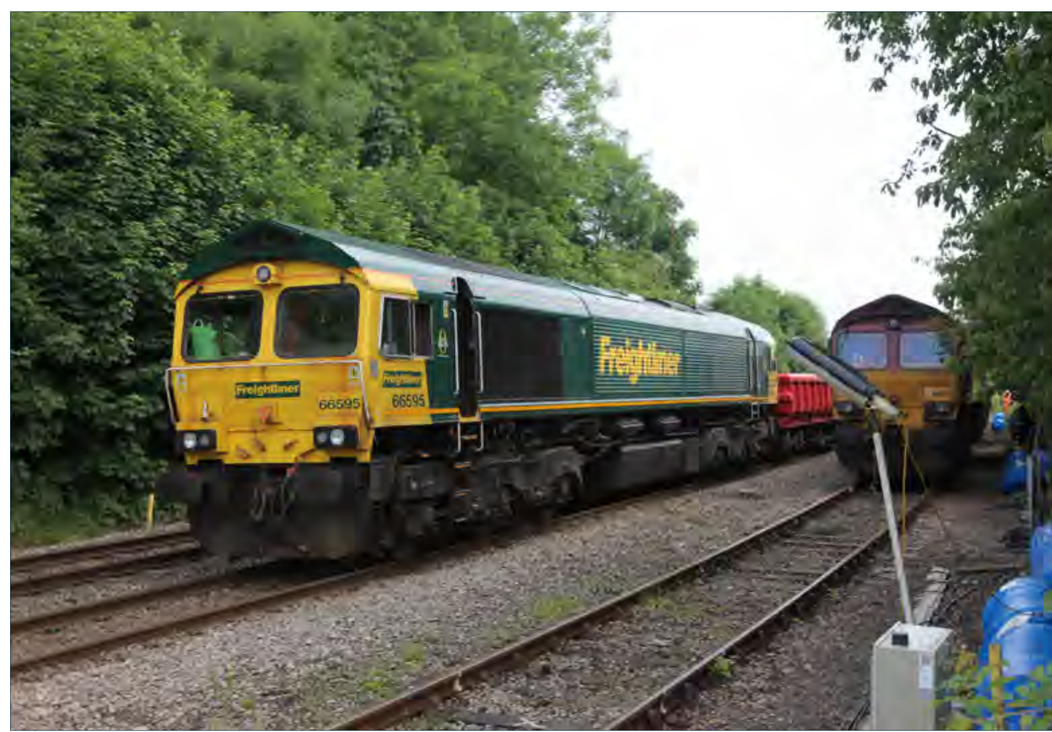
Class 66 595 and 66 047 are pictured at Malvern Wells during track re-laying works. Neil Pugh
