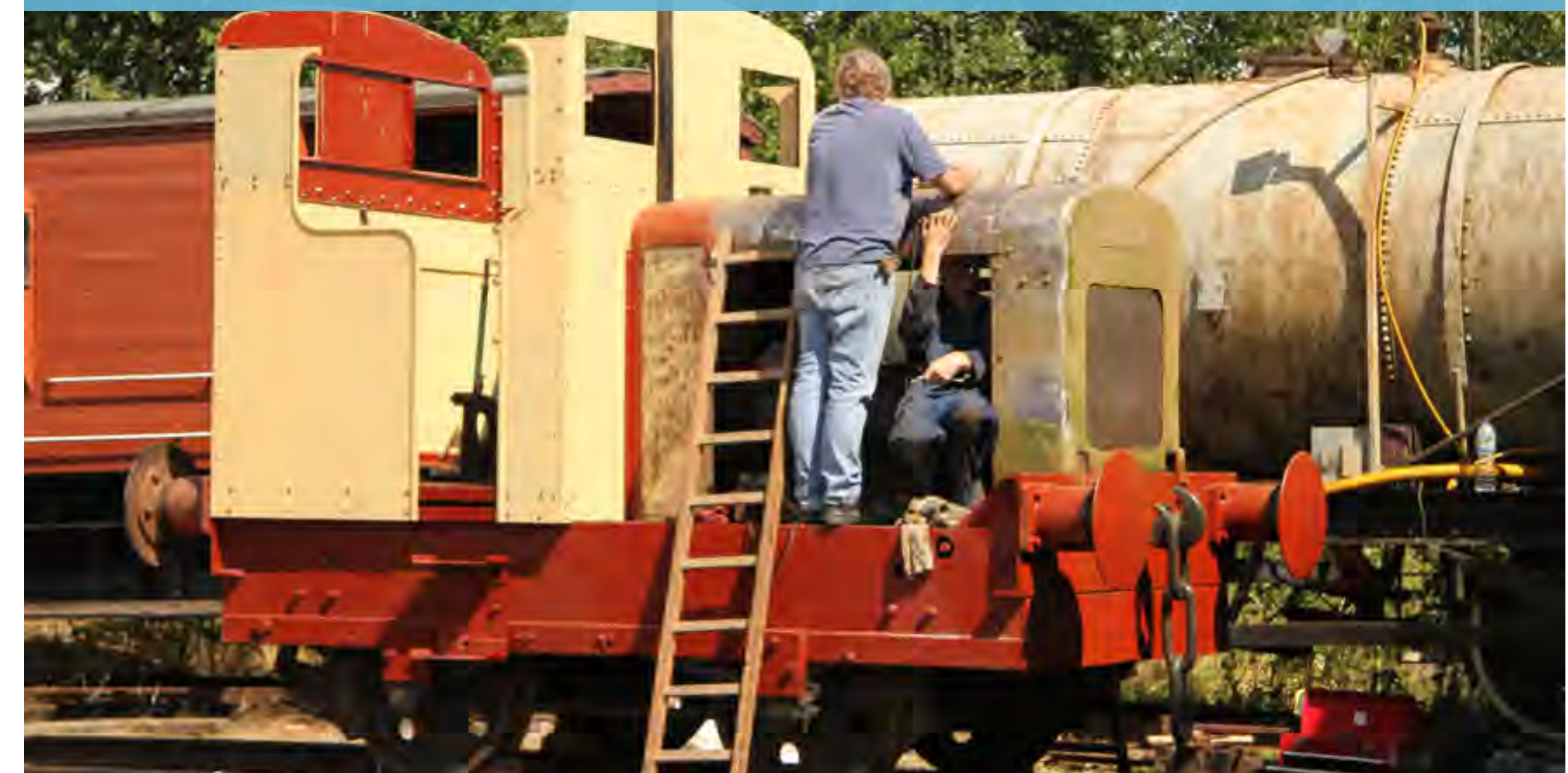
Ruston & Hornsby 88DS, works No. 207103, is another loco undergoing restoration at Cottesmore. Derek Elston
