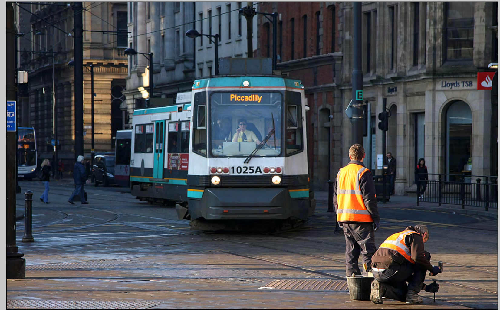
Above: With the workmen busy sorting out the paving, No. 1025 approaches Piccadilly Gardens. Derek Elston Below: Manchester Metro No. 3010 arrives into Piccadilly Gardens, on November 20th. Derek Elston
