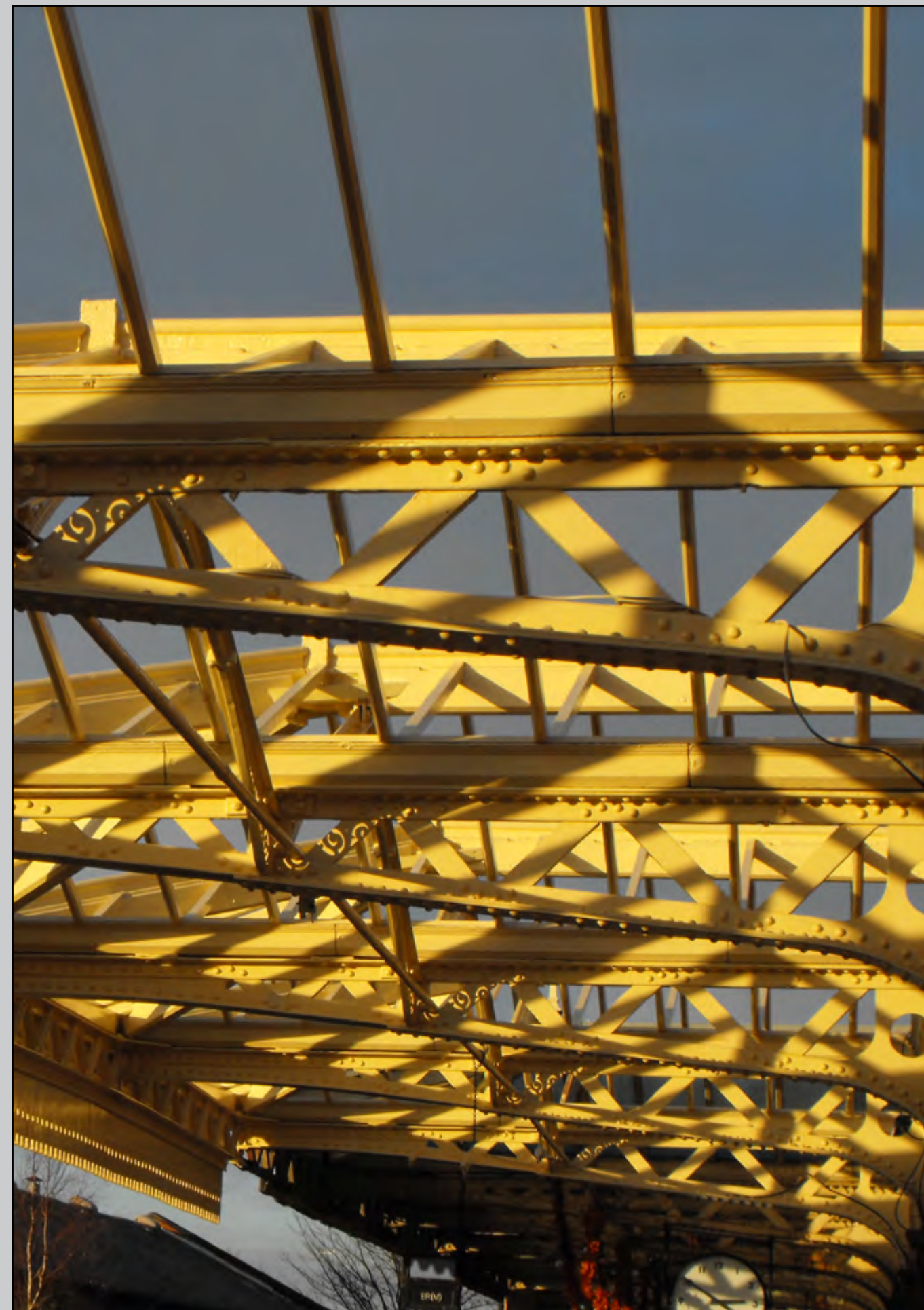
Photo: The sun illuminates the restored canopy on platform 2 in Jan 2012, awaiting the contractors to install the glass. © Tom Ingall
