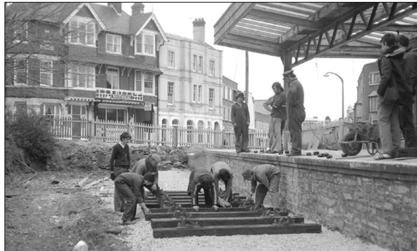
Photo: Swanage station track laying in 1977. © JOHN KELLAWAY courtesy SWANAGE RAILWAY TRUST
